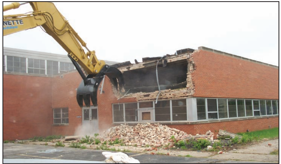
Principle Construction crushed and recycled the concrete and asphalt, and salvaged and resold the steel and brick on this Bedford Park redevelopment, resulting in cost savings and environmental benefits.
